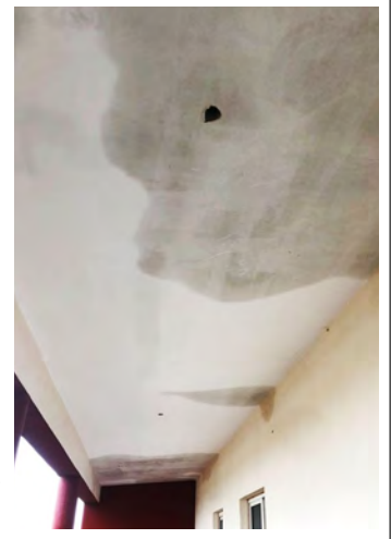
The torrential rain caused damage to the roof and water penetrated the masonry of our clinic. Now we have to repair the damage and the roof quickly.
